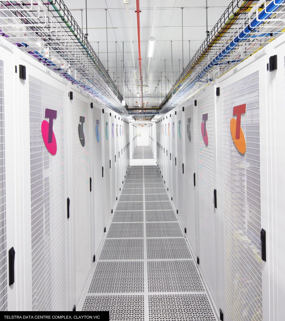
TELSTRA DATA CENTRE COMPLEX, CLAYTON VIC
