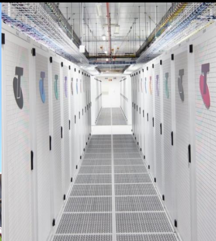
CENTURIA: TELSTRA DATA CENTRE COMPLEX, CLAYTON, VIC
